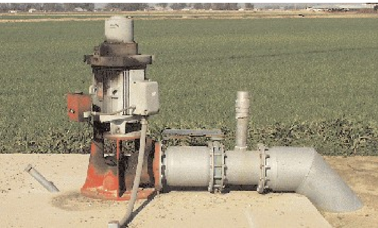
Properly completed well with elevated concrete seal (but with leaking lubricant).
