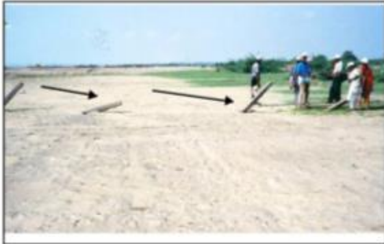
Deflected Pillars in Samiyapettai village (Nagapattinam area)
