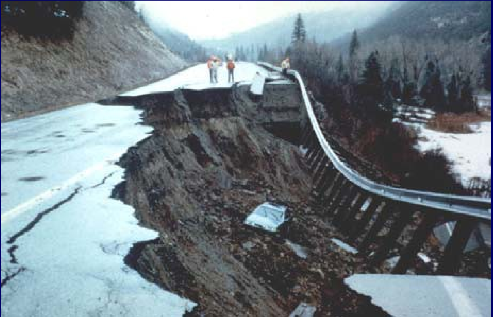
Slump in McClure Pass, CO.
